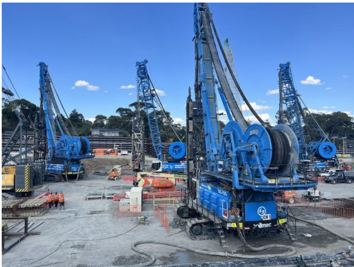
Four new Soilmec hydromills are excavating 90,000 cubic metres of soil and rock (Courtesy of Trevi)
